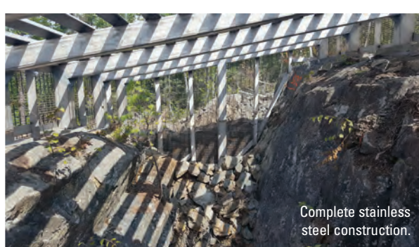
Completed Edison open cut cupola with bat-friendly 146-mm spacing between all steel members.
